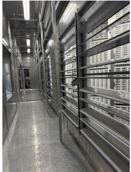
Large custom data center AHU
