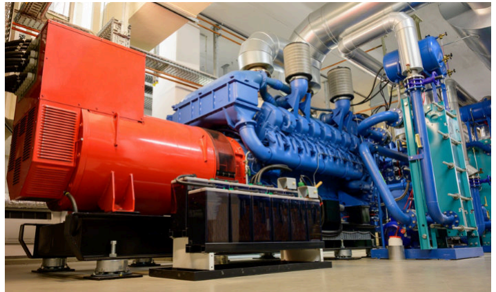
Large generator with paralleling gear
